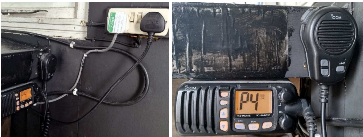
The VHF transceiver in the signal tower is an ICOM IC-M401E.
